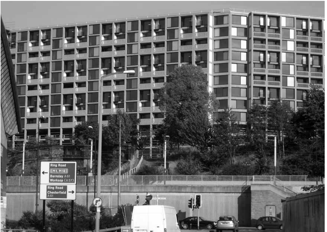
Figure 1. Park Hill under renovation, 2010. (Photo: CC ThomasB443) (Cladding from some of the Park Hill tower blocks has now been sent to the BRE for testing.)
