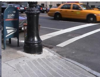
Scored cement, slab & asphalt
