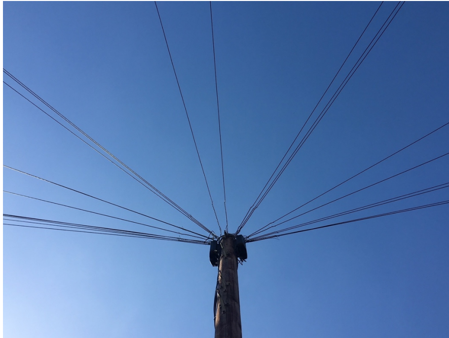
Figure 3.20. Telephone cable pole, London, 2018
