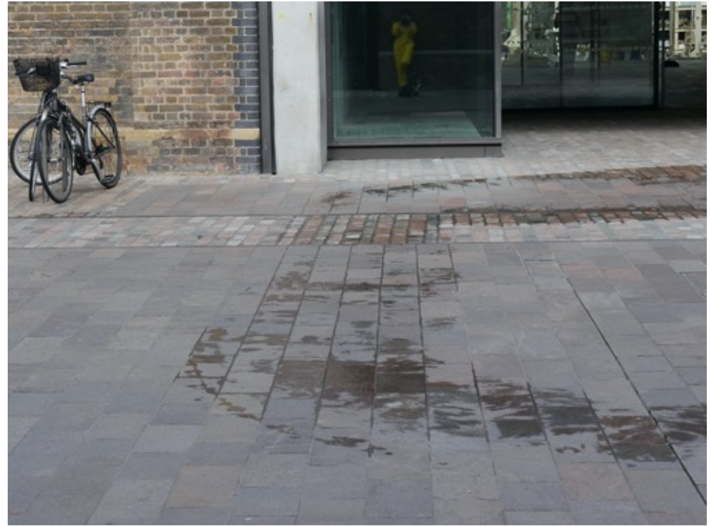
WATER TRACES LEFT BY RIDE-ON SWEEPERS. KING'S CROSS ESTATE. FIG. B01.
