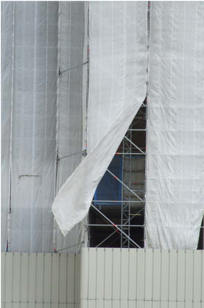
Fig.4 Covered scaffolding on the side of a building, Paris, 2012. Photo: Kim Bagley.
