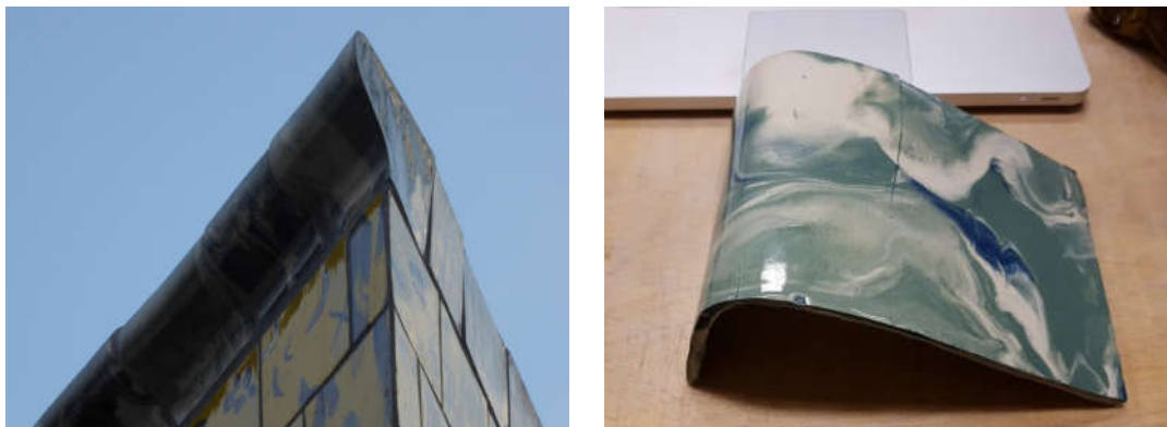
Fig. 3.7. Left: cornice formed by irregular hand-made tiles. Right: a cracked hand-made tile made by being slumped in the plaster mould (2017)
