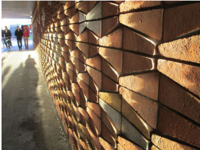
Fig. C.7. Humtunnel, Delft. Brick artwork three years after completion (2016)
