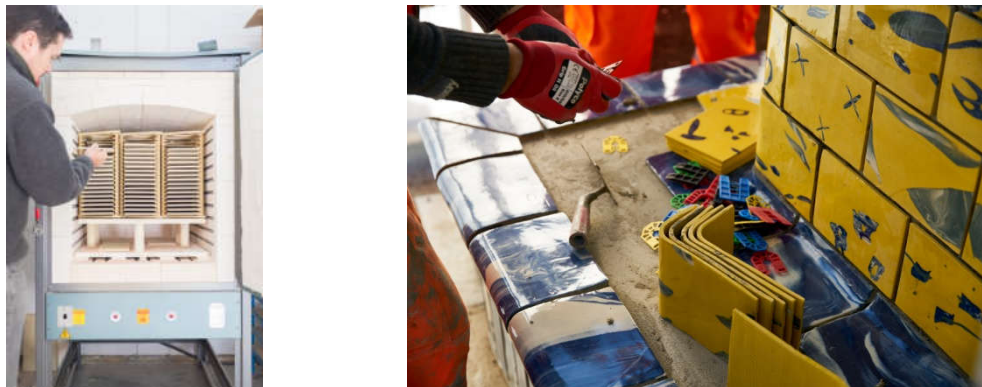
Fig. 3.8. Left: Matthew Raw filling up the kiln at the studio. Right: tiling contractors on site (photos: courtesy of Assemble, 2017)
