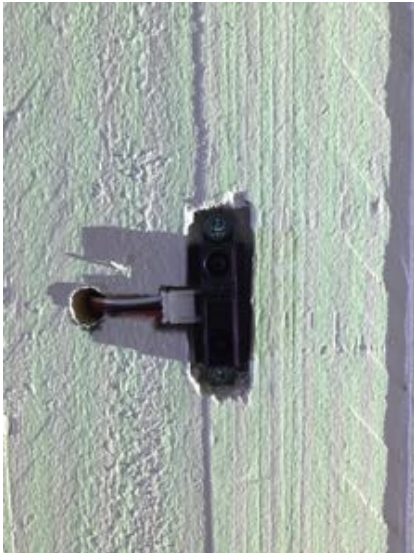
A Detector mounted into the wall
