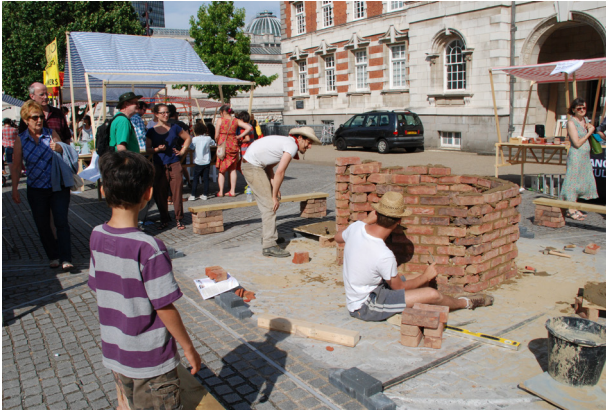
Figure 3.6: Pangaea Sculptors' Centre demonstrates bricklaying by building a tower inspired by the panopticon that once surveilled the area, when it was part of the Millbank Prison. Photo credit Marsha Bradfield.
