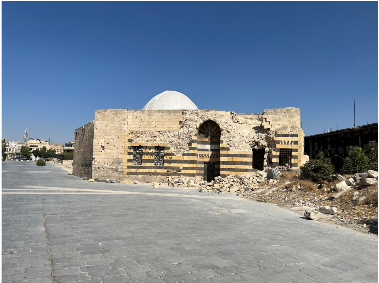
Fig 16. Hammam Yalbugha al-Nasiri , Earthquake destruction. Aug 2023. Digital photograph: Sally Hilal.
