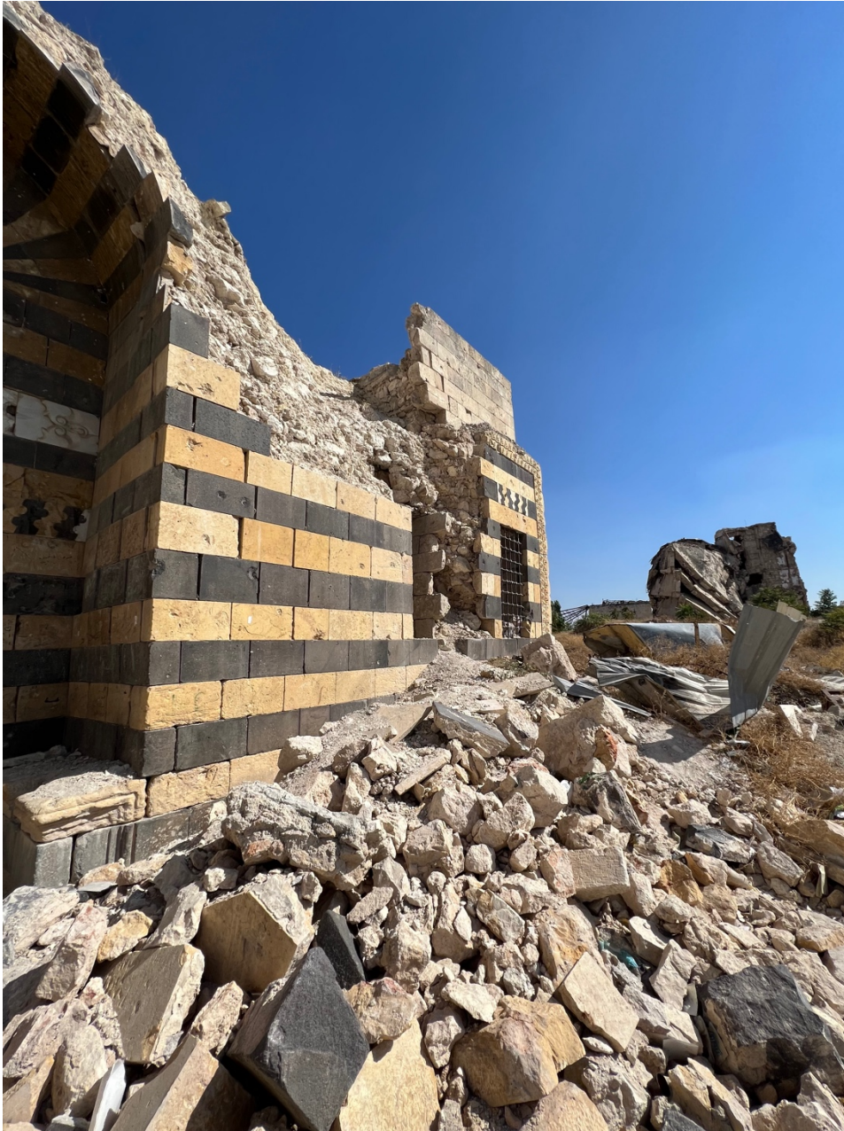
Fig 62. Hammam Yalbugha al-Nasiri, Earthquake destruction. Aug 2023. Digital photograph: Sally Hilal
