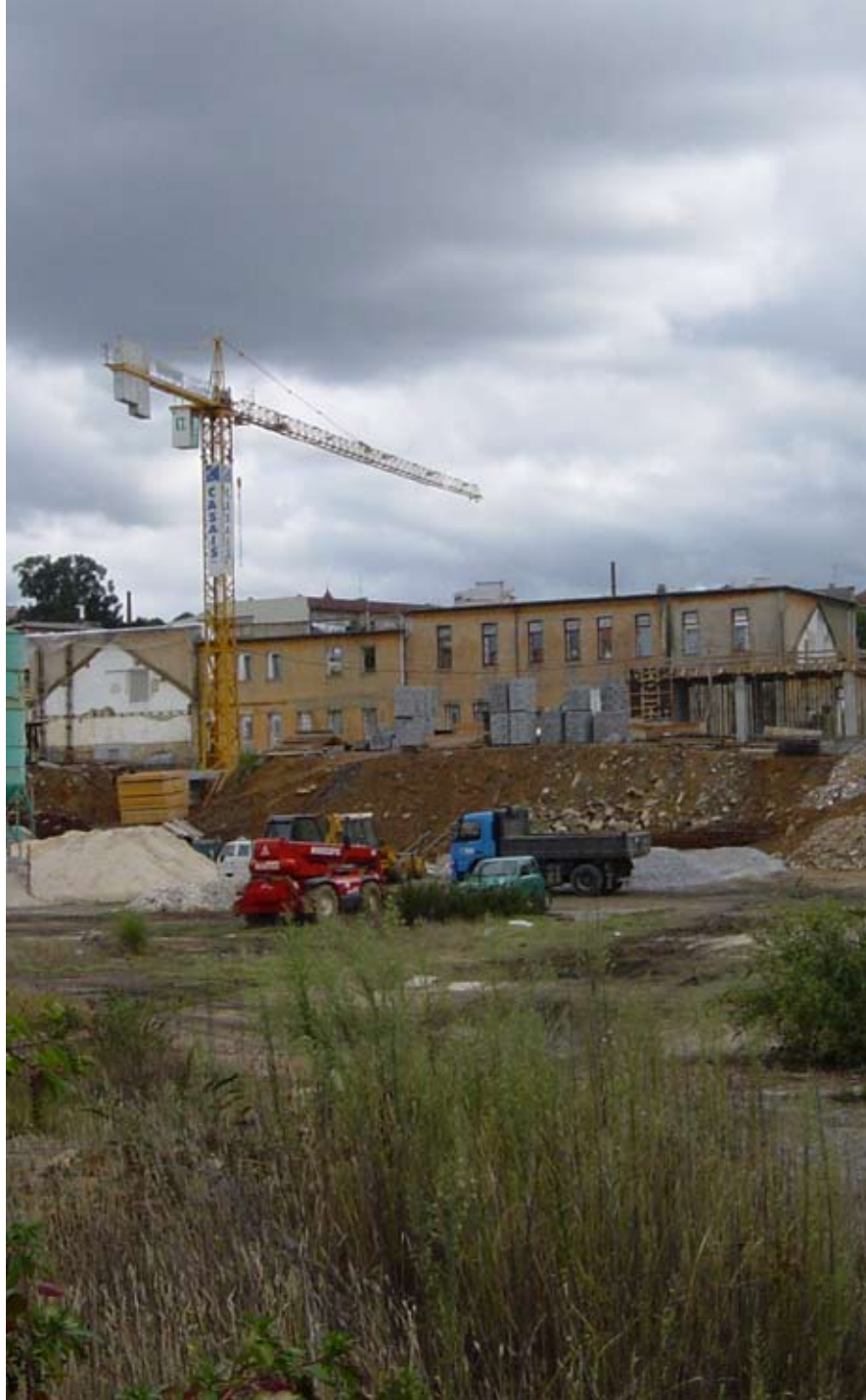
Construction of the Museu da Chapelaria on the former site of the Empresa Industrial de Chapelaria, S. João da Madeira, 2003. Photograph courtesy of Daniel Regalado Neto.
